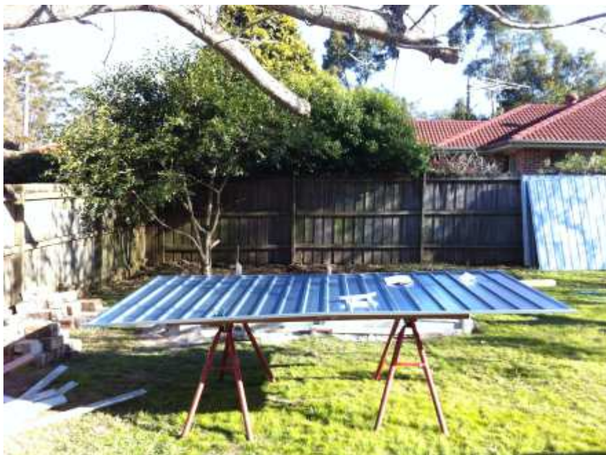
Figure 29.: Monday afternoon 3:39pm – last side panel, other walls are leaning against fence
