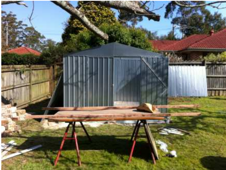
Figure 31.: Tuesday afternoon 2:24pm – how am I going to install the roof panels?
